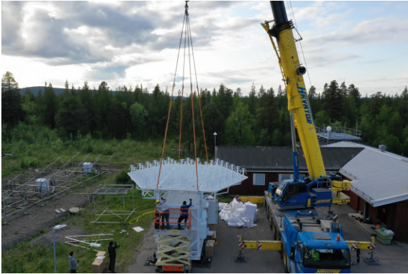
Figure 1: PET AU Installation in Kiruna.
